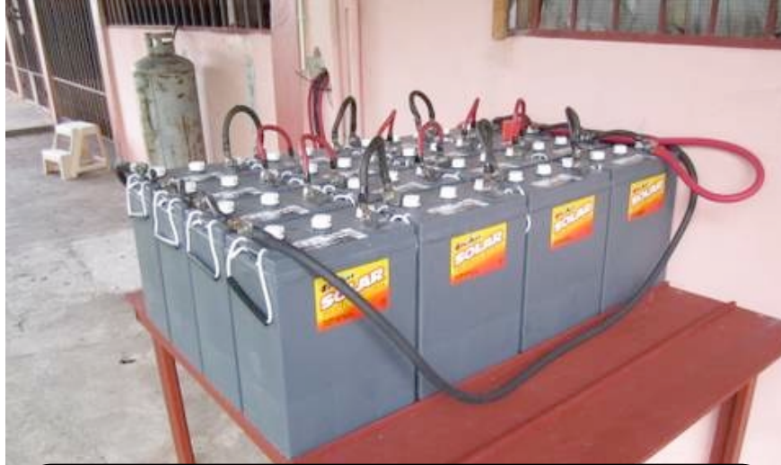
Our new batteries on the new battery table. We left room for 12 more batteries in the future.
